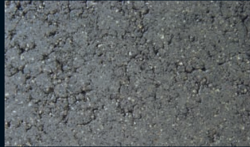
FISSURED AC F01
