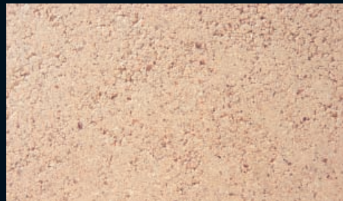
FISSURED AC F10
