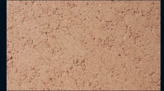
FISSURED AC F03
