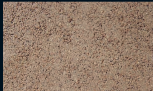
FISSURED AC F07
