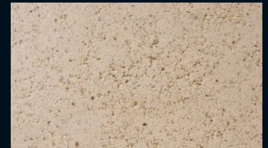
FISSURED AC F12
